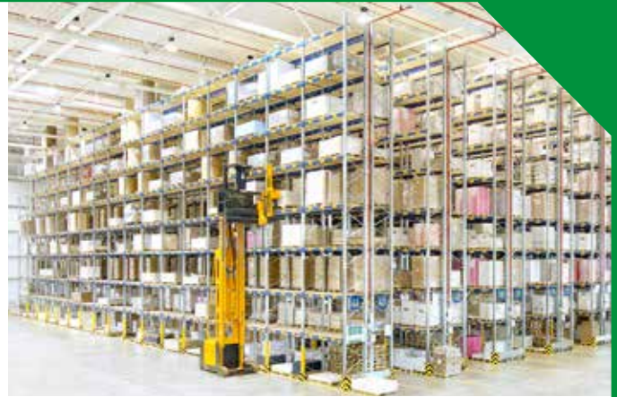
High-bay pallet racking
