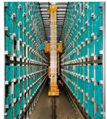
Storage & retrieval machine (SRM)
